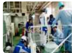
Pump piping line check
