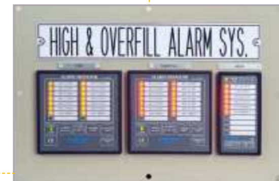
High & Overfill Alarm Unit
