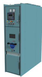
AMP Incoming Panel
