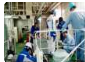
Pump piping line check
