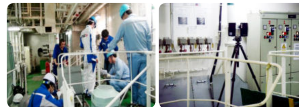
Pump piping line check
