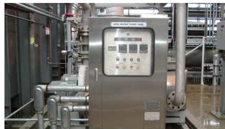
Local Control Panel
