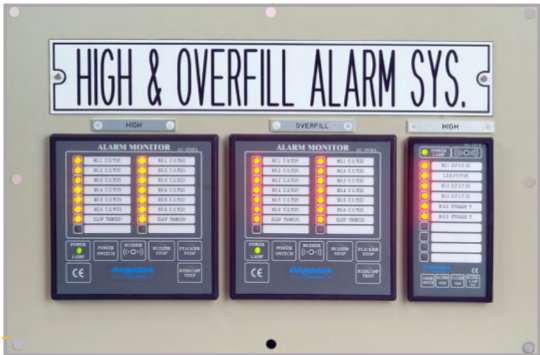
High & Overfill Alarm Unit
